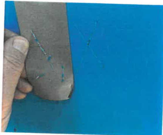
PHOTO #4: Adhesion test north side of riser.
